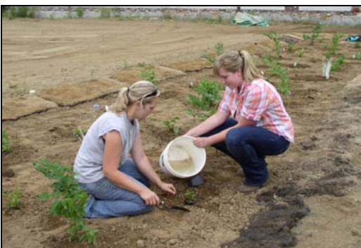
June 7th - Kayla Finton (R), NRCS Summer Intern, and Mary Thomas, SWCD Administrative Assistant, complete the planting of the Rain Garden at the Pomerene Center for the Arts former Park Hotel lot on Main Street. Special thanks to The Garden Patch Greenhouse and Roscoe Village Landscaping Department for their donations of plants.
