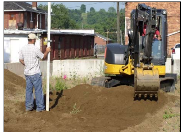
June 6th - SWCD Technician Ryan Medley checks grade as Steve Hubble from William Albert Inc. completes digging of the Rain Garden at the Pomerene Center for the Arts former Park Hotel Lot. Special thanks to William Albert, Inc. for donating their time and services to this project.
